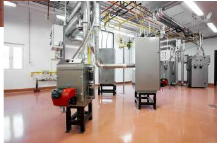
Bio oil and bio gas burner laboratories
