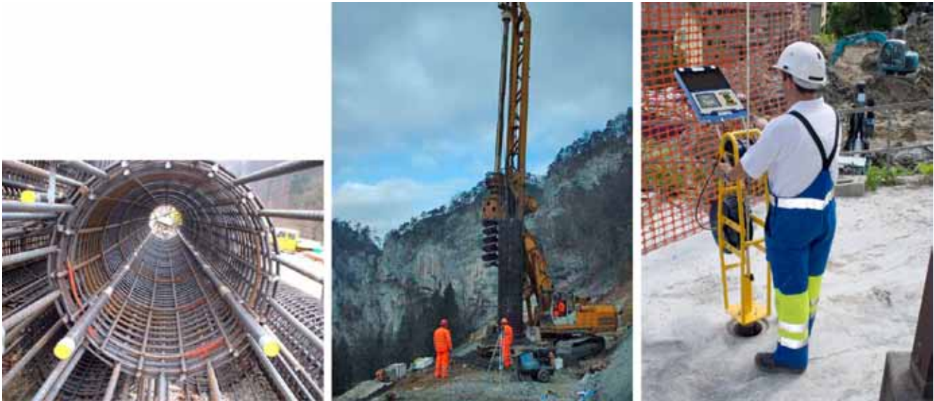
Figure 5 left: Pile reinforcement equipped with Trivec, Figure 5 center: Installation of reinforcement, Figure 5 right: Measurement with the Trivec
